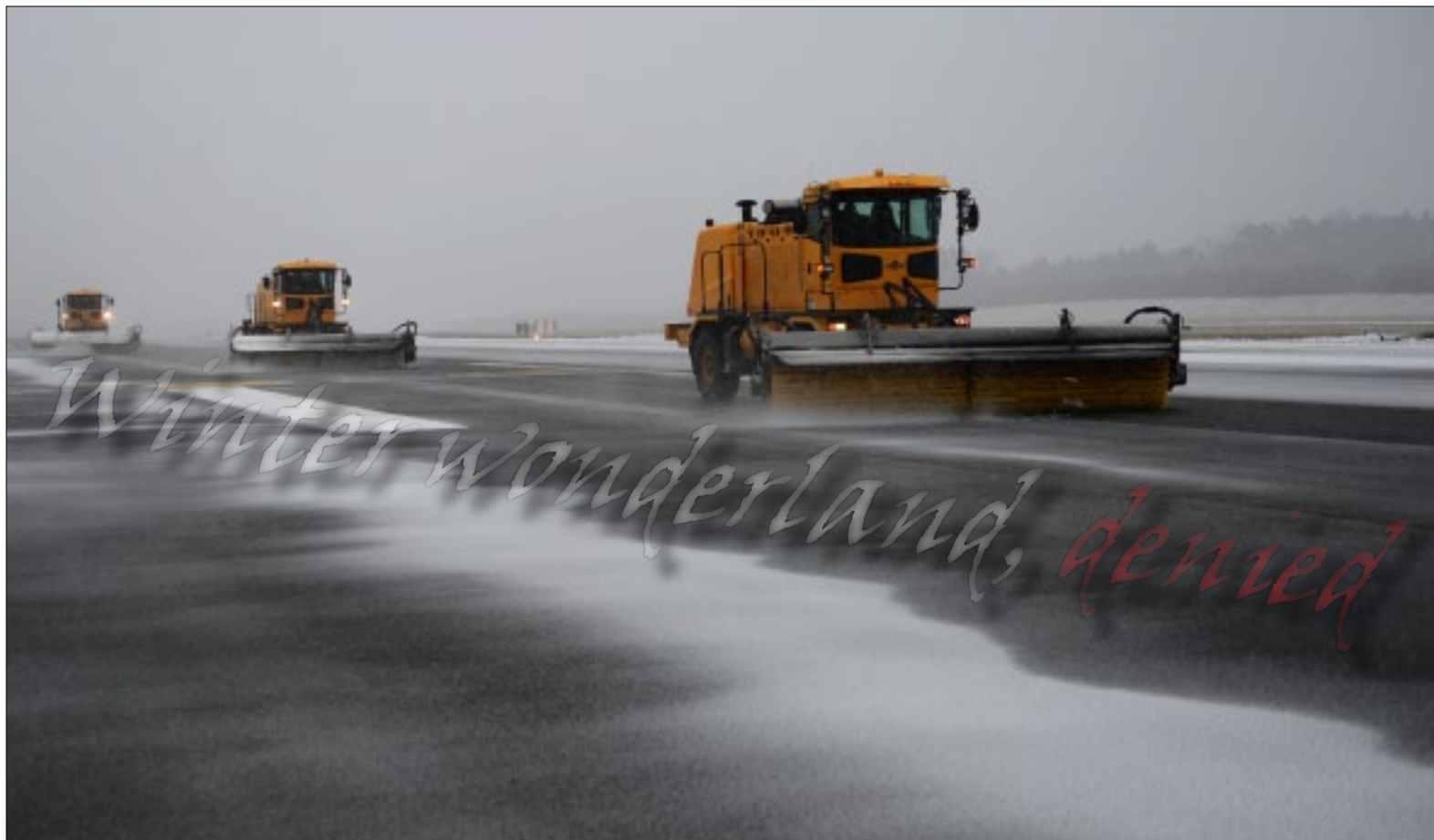
Members of the 52nd Civil Engineer Squadron snow patrol clear the flight line using vehicles such as a snow broom truck after the first snow of the season. The 52nd CES pavement maintenance and heavy equipment shop augments more than 30 Airmen each year to ensure Spangdahlem personnel continue to meet mission requirements. View more photos at http://www.spangdahlem.af.mil/news/story.asp?id=123328531 . (U.S. Air Force photo by Airman 1st Class Dillon Davis/Released)
